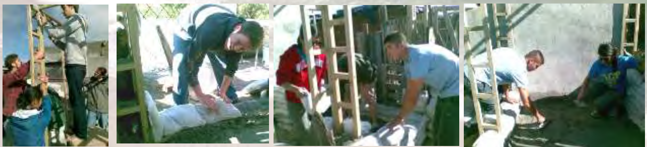
ABOVE: This is the stage where the actual construction of building and the laying of the sandbags begins...
